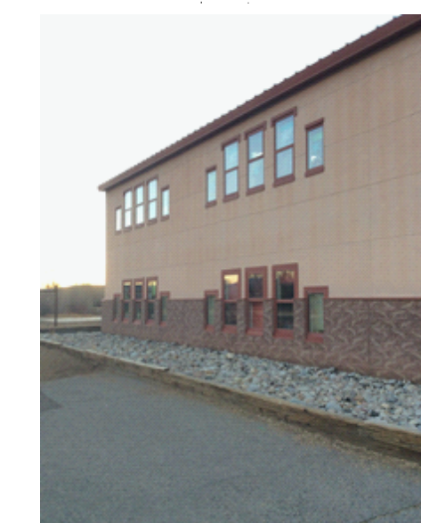
Windows are starting to leak according to maintenance
