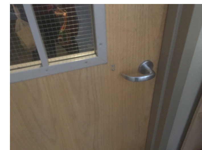
Door hardware is ADA compliant, but not code compliant
